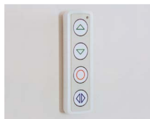
Wireless landing controls
